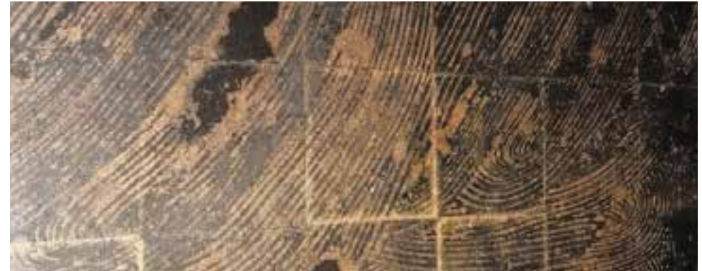
Asbestos bitumen adhesive use to stick floor tiles down
