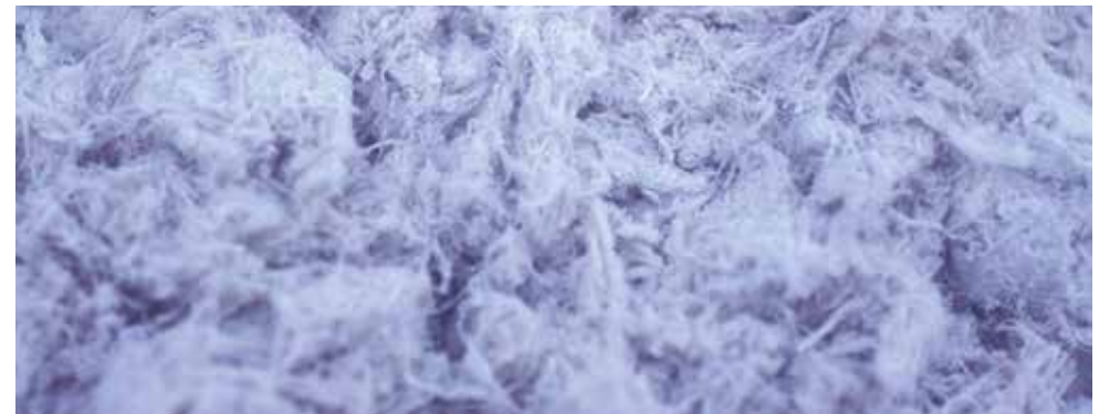
Loose fill blue asbestos from a wall cavity
